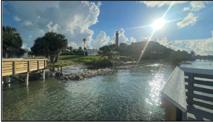
Photo 3: View of recently constructed living shoreline at the Jupiter Inlet Lighthouse Outstanding Natural Area
